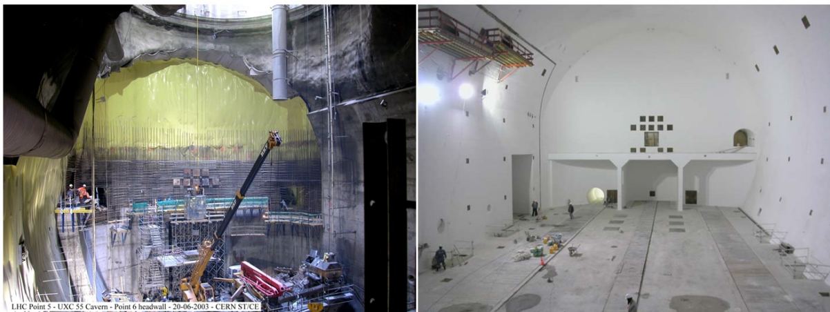
Figure 76: The construction of the CMS cavern for the LHC project at CERN, Geneva.
